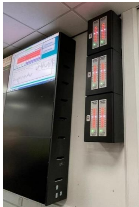
Remote Indicating LEDs in the Control Room Prior to Start-Up
