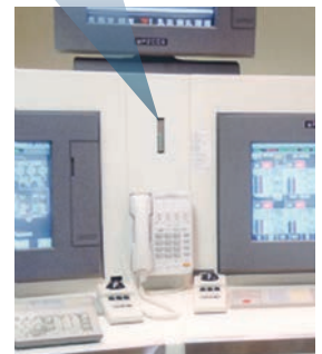
SIS Indicator in control room.
