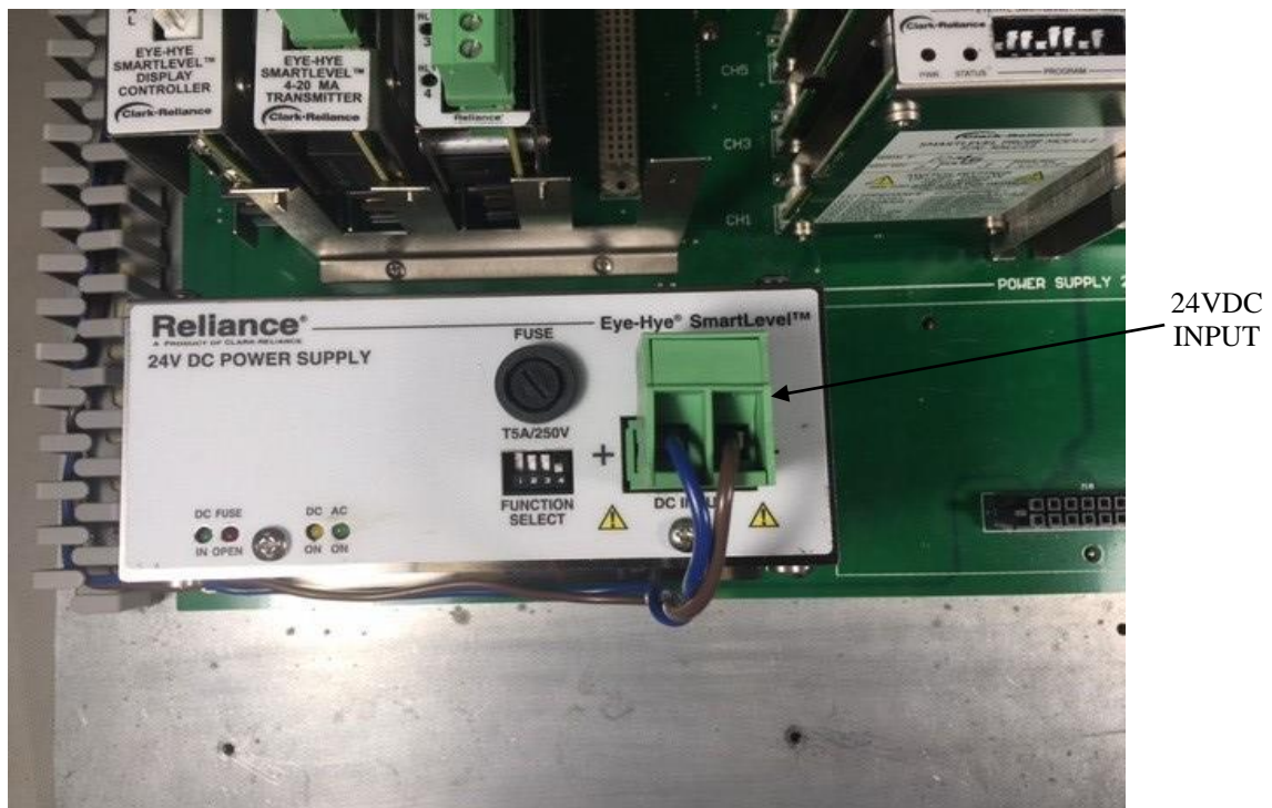
FIGURE 3 – Standalone RSLC91 24VDC Power Supply in POWER SUPPLY 1 position
