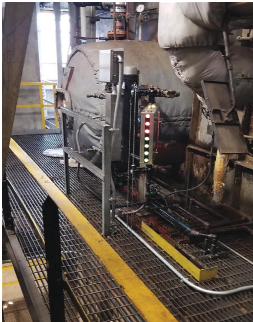
FIGURE 1. A ported-type water gage installation with properly installed illumination accessories. Image courtesy of Clark-Reliance
