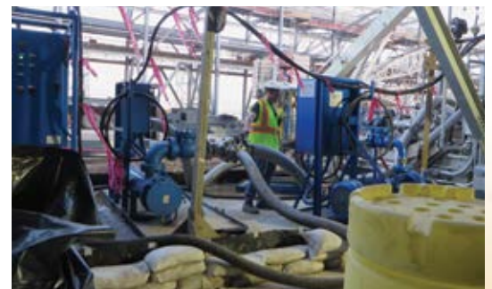
Compressor Lube Oil System commissioning High Velocity Oil Flush at a LNG plant in Louisiana
