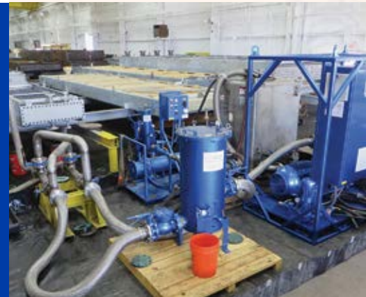
High Velocity Oil Flush of cooler bundles at a manufacturer's plant in Houston, Texas
