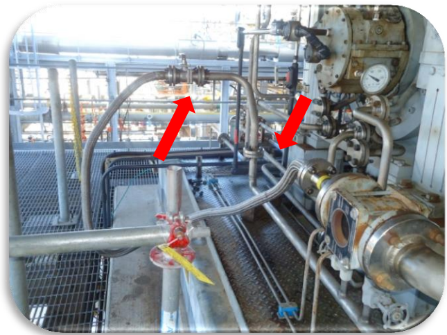
Jumpers Installed On Lube Oil Piping
